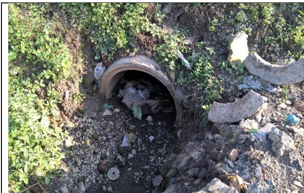
Debris found in the storm water line
