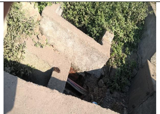
Broken Storm water line
