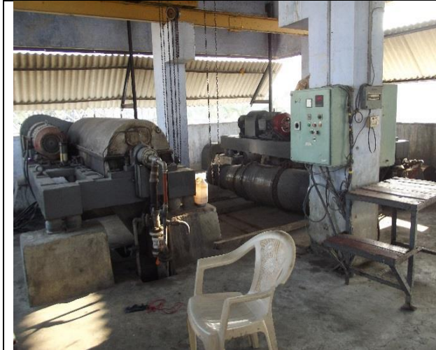
Decanters for Sludge de-watering
