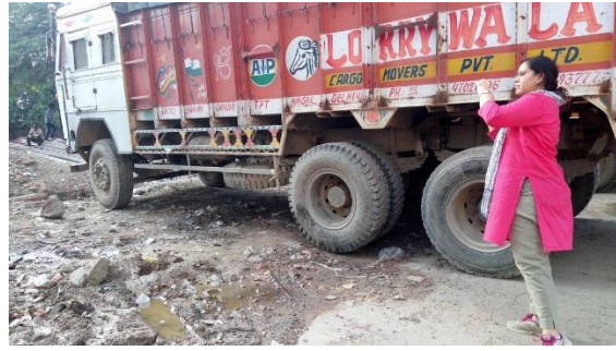
Broken road and water logging problem during monsoon in Lawrence Road Industrial Area.
