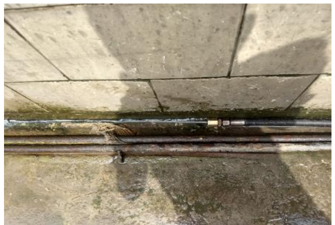
Pic 2: Measure 1: „After“ Closed hose
