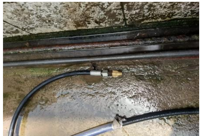
Pic 1: Measure 1: „Before“ Open hose in the car washing industry
